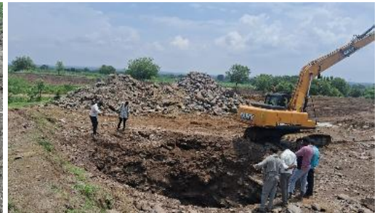
Community Irrigation Well At Balewadi
