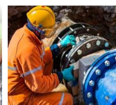
Operations and Management Of Community Water Supply
